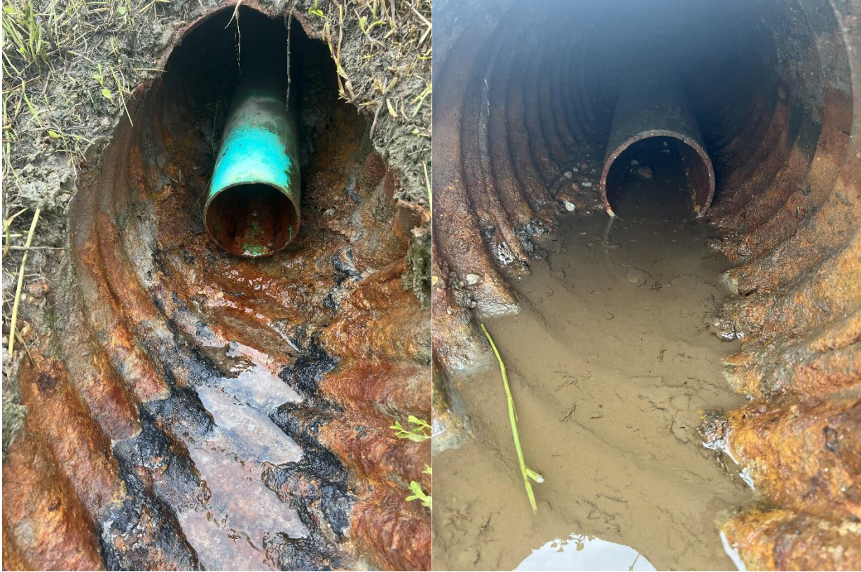
Figure A3. CCR Landfill Cell 1 (Left) and Cell 2 (Right) Underdrain Outlet; 7/10/2023
